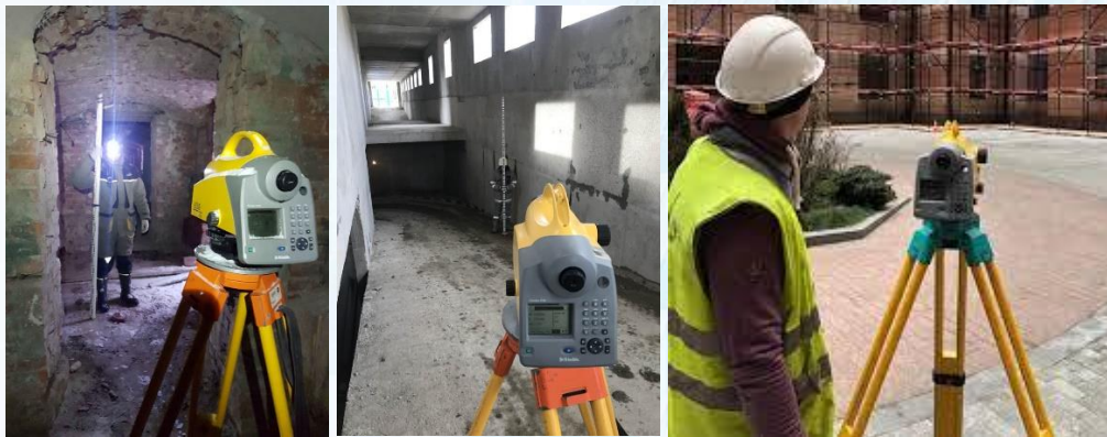
Figure 4. When monitoring the deformation of the building and structure used digital levels
